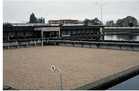
Clean slow sand filter without water layer
