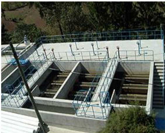
Rapid Sand Filter
