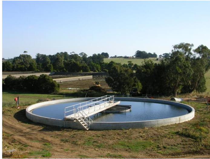
A photograph of circular sedimentation tank
