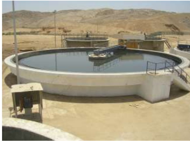
Primary sedimentation tank (Radial flow)
