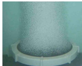
Diffused air system of aeration tank
